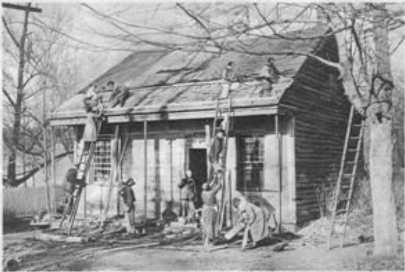
A shingle bee. To save face and their town's claim to fame, residents of Ralston, N. J., pitch in to recondition the dilapidated post office – one of the nation's oldest. Crisis was precipitated when Mrs. Catherine Groenewegen, postmaster, moved office from the historic structure because she "well nigh froze to death in it."
