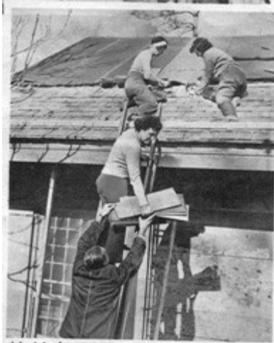
Municipal enterprise. John H. N. Potter and Mary Langford pass shingles up to Mrs. Margaretta Potter (left) and Mrs. Florence C. Page, who fix new roof. Residents have organized Ralston Historical Association to restore the post office landmark. Sunday Evening January 11, 1942
